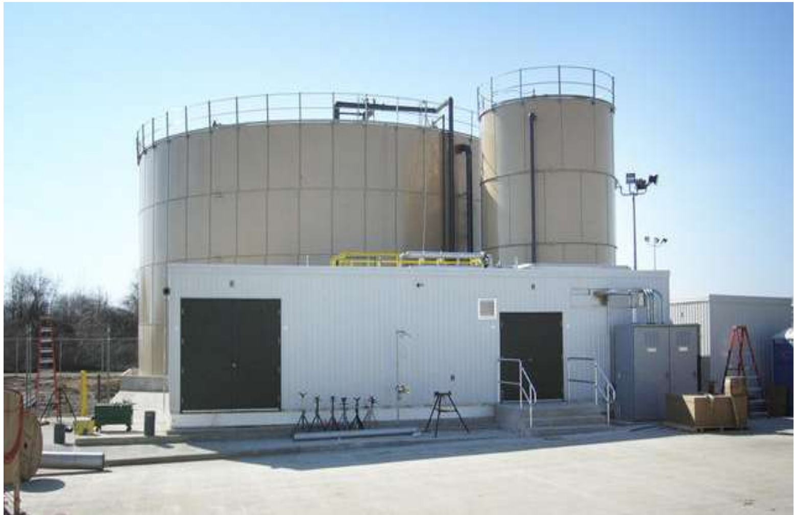
Membrane Bioreactor System
