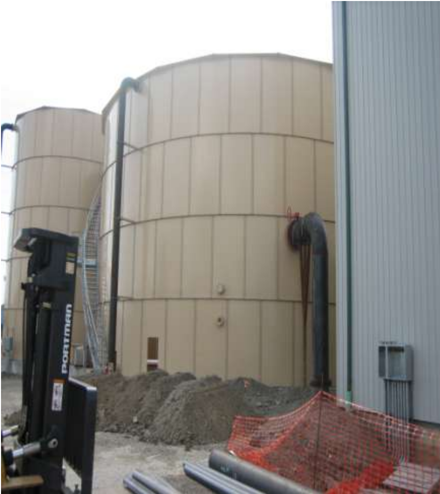
Anaerobic and Aerobic Bioreactor Tanks
