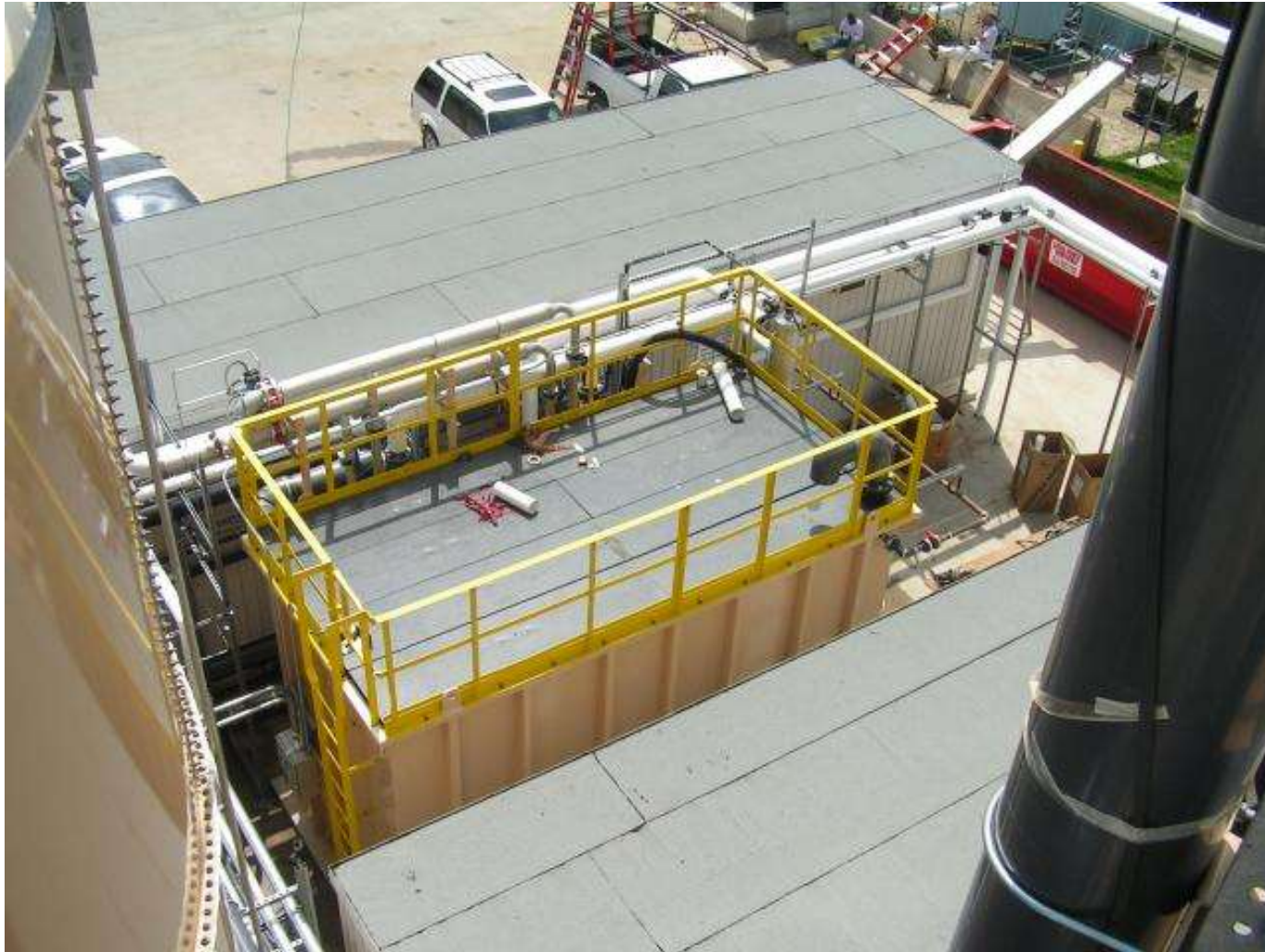
Steel (Above Ground) Membrane Tank
