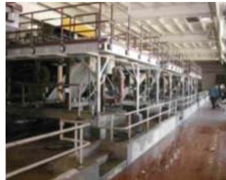
Belt Filter Presses
